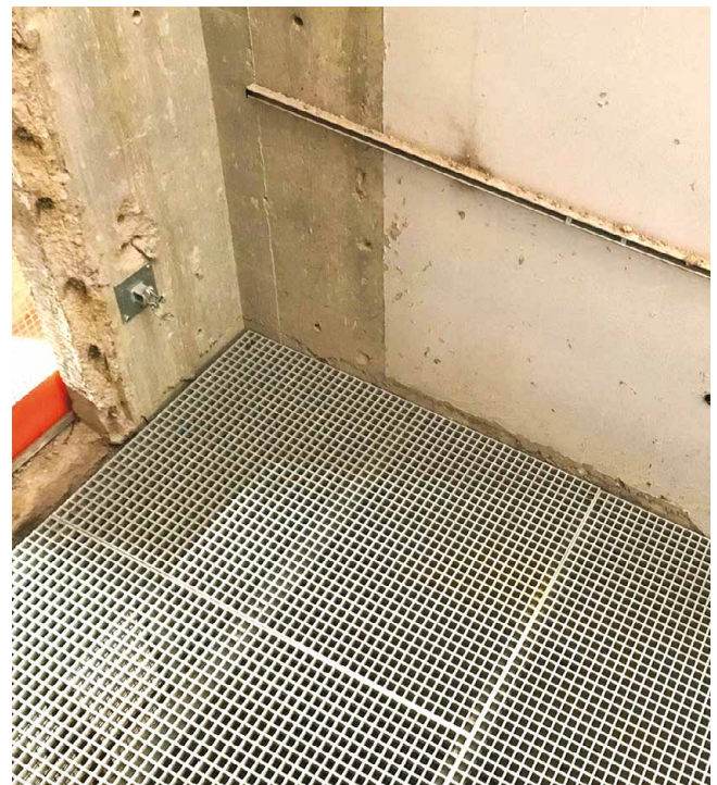
Riser Floor fitted at required floor datum height, ready for service penetrations.
